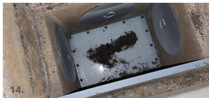
The clean-outs are located under the ash box.
